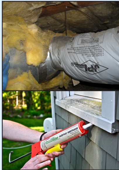
Adding insulation and sealing ducts and home openings can make a big difference.
