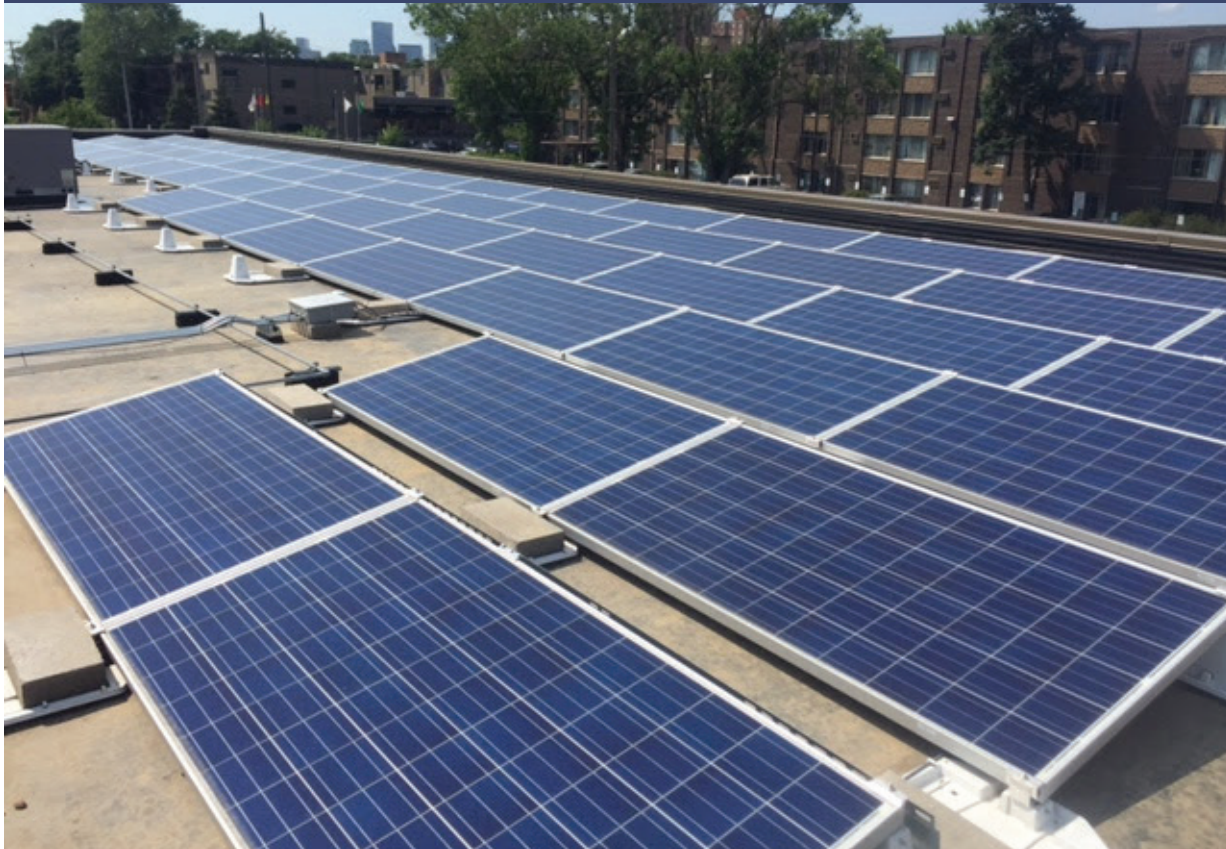
Solar panel installation on the roof of 2327 E. Franklin Avenue. Photo Credit: Joshua Houdek
