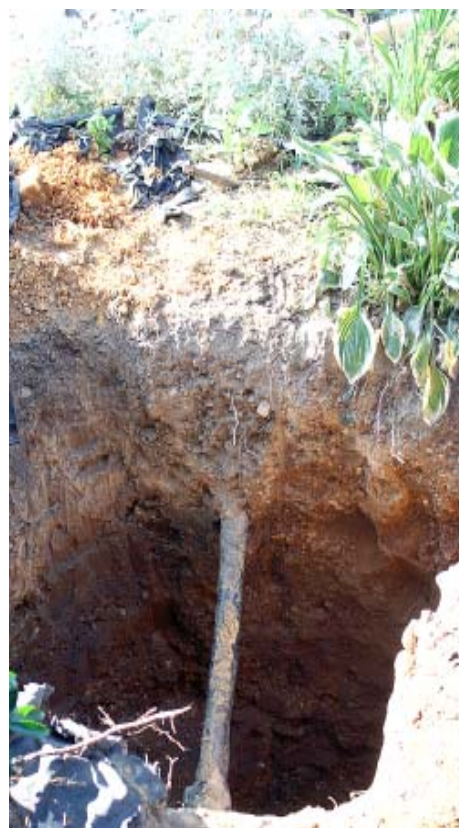
Lead pipe cinch A lead water main in Washington DC
