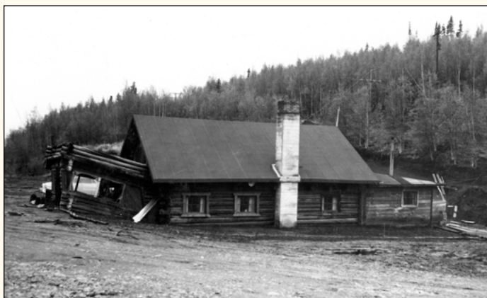
Roadhouse, mile 278.5, Richardson Highway. The structure is distorted because of thawing of the underlying ice-rich permafrost in fine-grained silts and sands. Gulkana district. Copper River region, Alaska, May 29, 1962. (Photograph by T.L. Pewe) Published as figure 33 in U.S. Geological Survey Professional Paper 678, 1969. Reprinted with permission.
